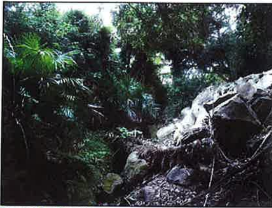
Figure 13 - Degraded drainage line from Burran Ave, with native palms Livistona australis
